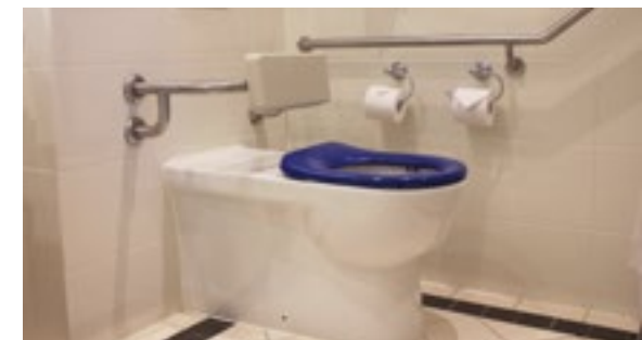
The bedroom toilet has grab rails, backrest, contrasted seat and emergency call.
