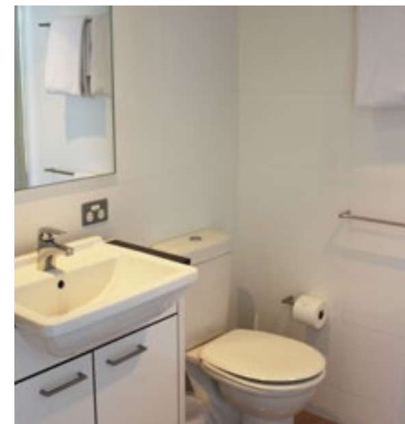
The bathroom design doesn't include grab rails.
