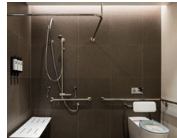
Roll-in shower, shower chair and accessible toilet with grab rails.
